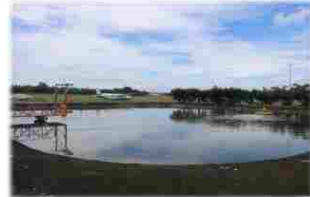
Wastewater treatment facilities
